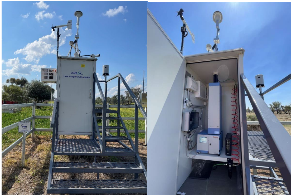
Figure 1: TEOM installed at Lanreef
